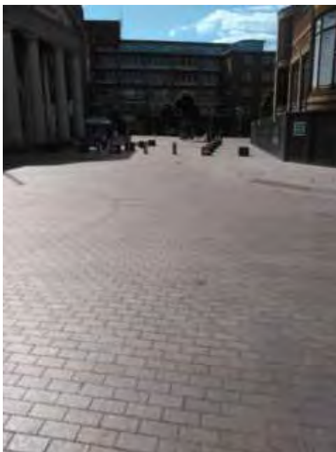
Photo 2: Shared space junction in Coventry illustrating potential trip hazards in the pavement area.
